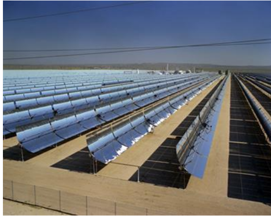
Solar electricity production (Photo: energy.ca.gov)
